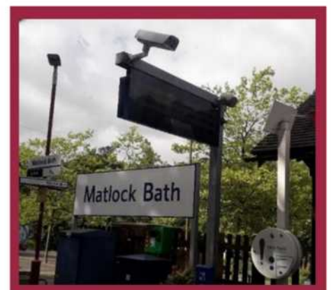
New CCTV at Matlock Bath
